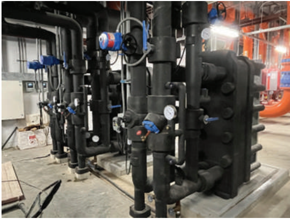
Energy Transfer Station (ETS)
